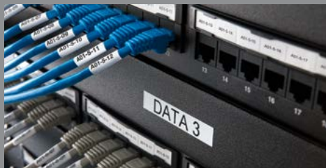
Wire & Cable Identification
