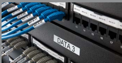
Wire & Cable Identification
